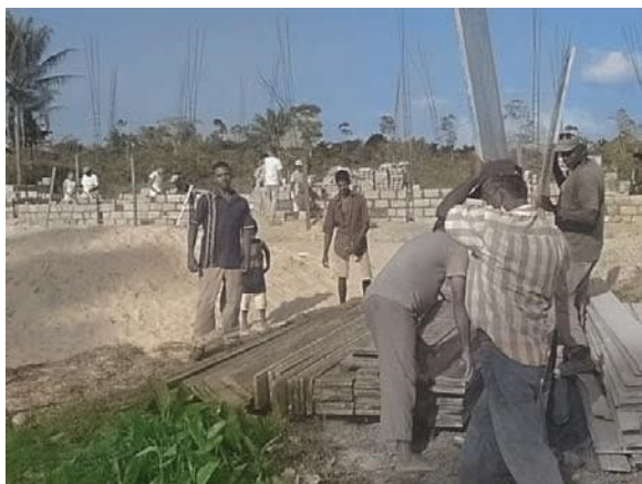
Construction goes forward on the school buildings at Kimbia Mission Academy as local individuals work with student missionaries from the United States to complete the needed facilities.
