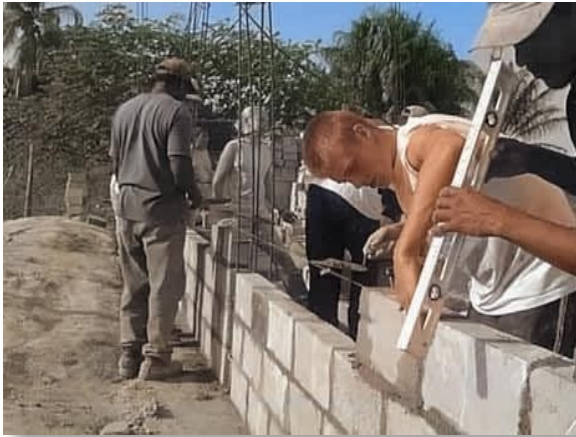
Work progresses on the initial school building at Kimbia Mission Academy. Here God performed a miracle with gravel!
